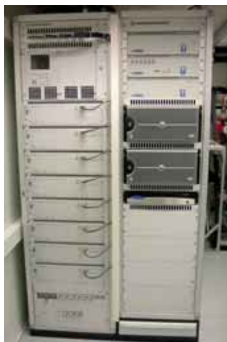
Transmit and receive control unit at the equipment shelter.
